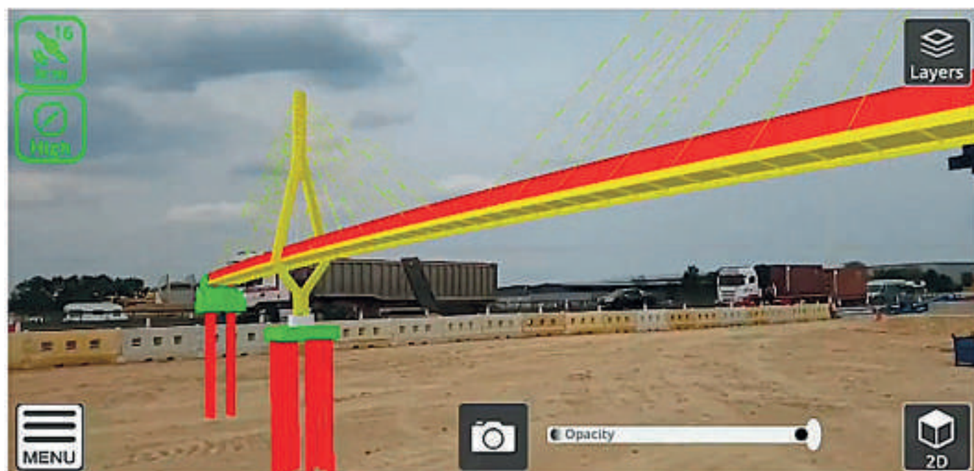
Trimble SiteVision: a fast, friendly way in which Augmented Reality can be exploited to share construction site information
