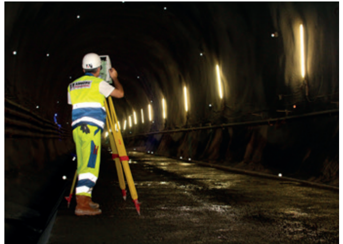
The surveyor measures convergence points to analyse the displacement of the tunnel surface
