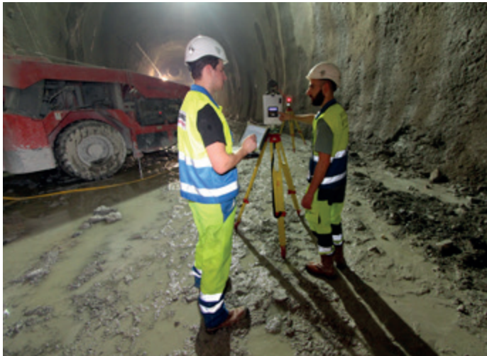
Laser scanner measurements with TMS Tunnelscan in front of the tunnel face to determine the complete information of as-built control
