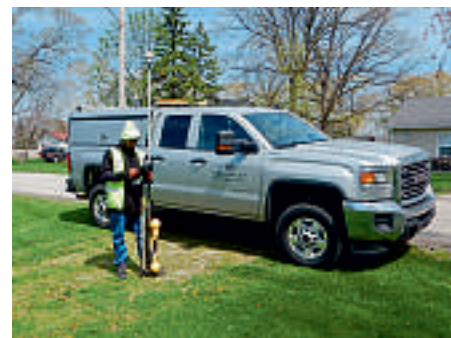
Vincent Johnson collects data above a gas pipeline. The system uses GNSS to produce georeferenced location and depth for the buried pipe
