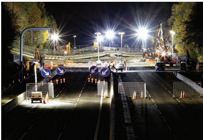
Smart Motorways, such as that currently being engineered between Junctions 2 and 4a on the M3 (pictured) will increasingly utilise telematics to optimise traffic flows. Photo: Highways England
