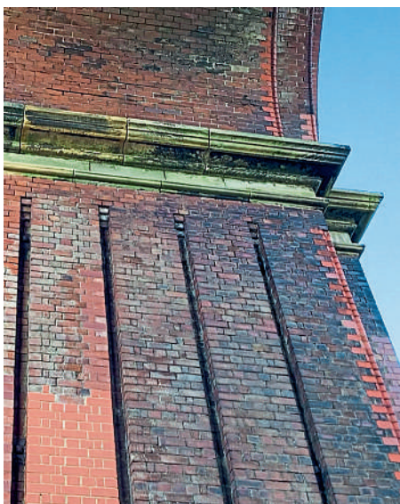
Seven million bricks and 436,000 cubic feet of stone were used in construction of the viaduct. It underwent a major renovation in 2016 when the arches were strengthened with 2,800 steel brackets and a new drainage system was installed at ground level in a bid to prevent flooding
